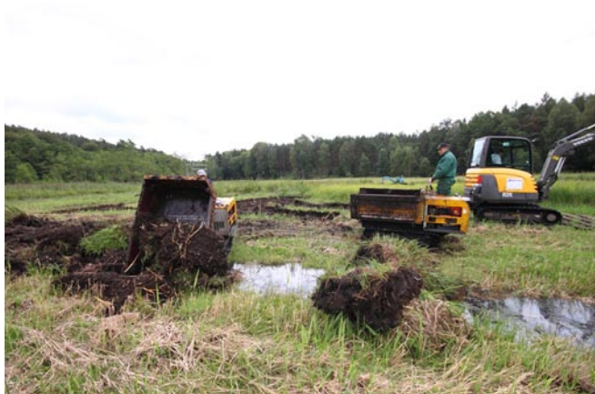
Fig. 1: Small track dumpers pour removed top-soil layer into the drainage ditches. Photo: Stiftung NaturSchutzFonds Brandenburg.
